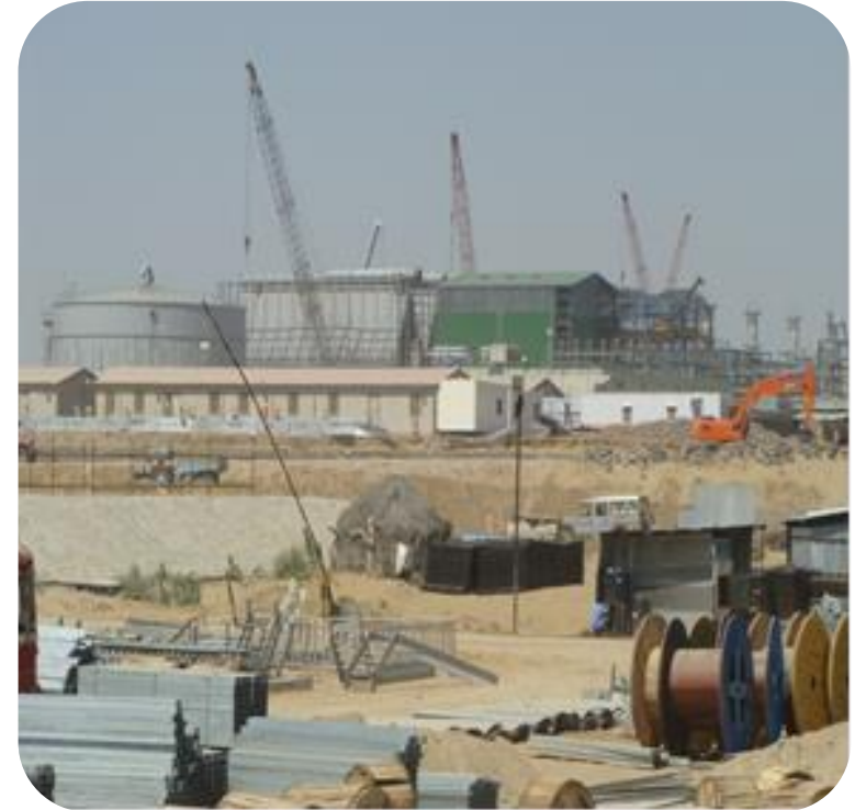
Photograph of Mangla Processing Terminal taken by Research Team
