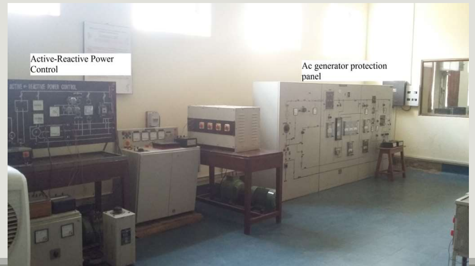
Power System Lab.
